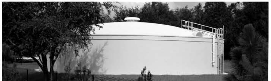
SUGARLOAF MOUNTAIN, LLC 0.5 MG WATER STORAGE TANK CONSULTING ENGINEERS: BOOTH, ERN, STRAUGHAN & HIOTT, INC.
